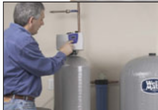
Installing a water softener system with a Fleck 7000 valve delivers the highest flow rates available in a residential system.
